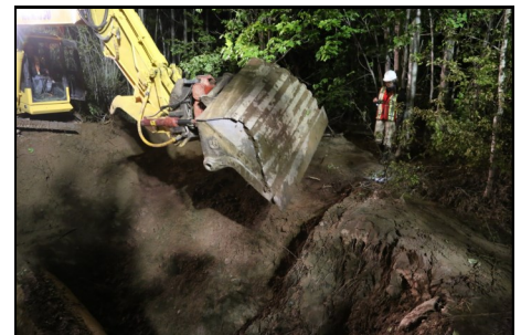
Photo above: Night time Monitoring of excavation to ensure no threats to burial locations
